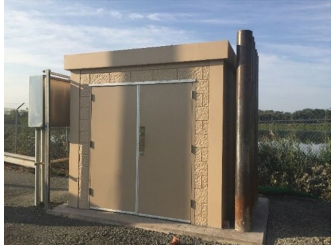
Onsite flood-resistant enclosure & bollards on concrete foundations
