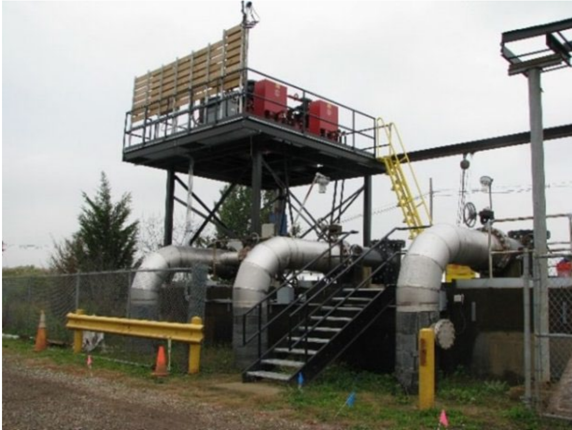
Elevated electrical controls for full-scale groundwater extraction
