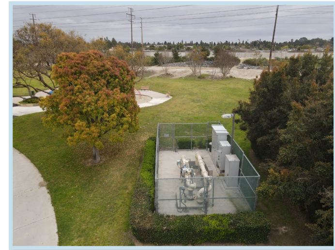
Aquifer Replenishing Well
