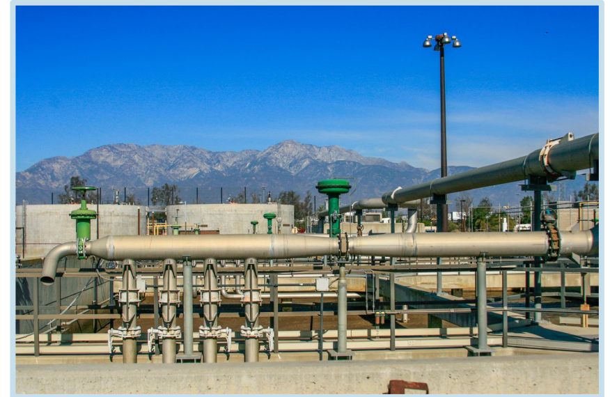
IEUA Regional Water Recycling Plant No. 1 Pipelines
