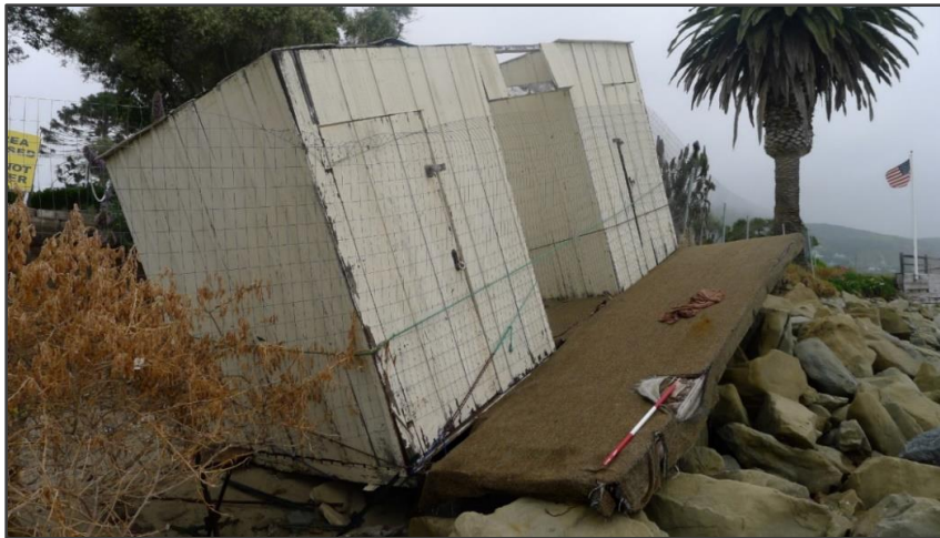
April 2019. Bathhouse undermined.
