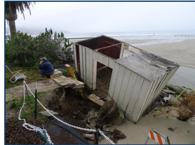
November 2019. Bathhouse eroded
